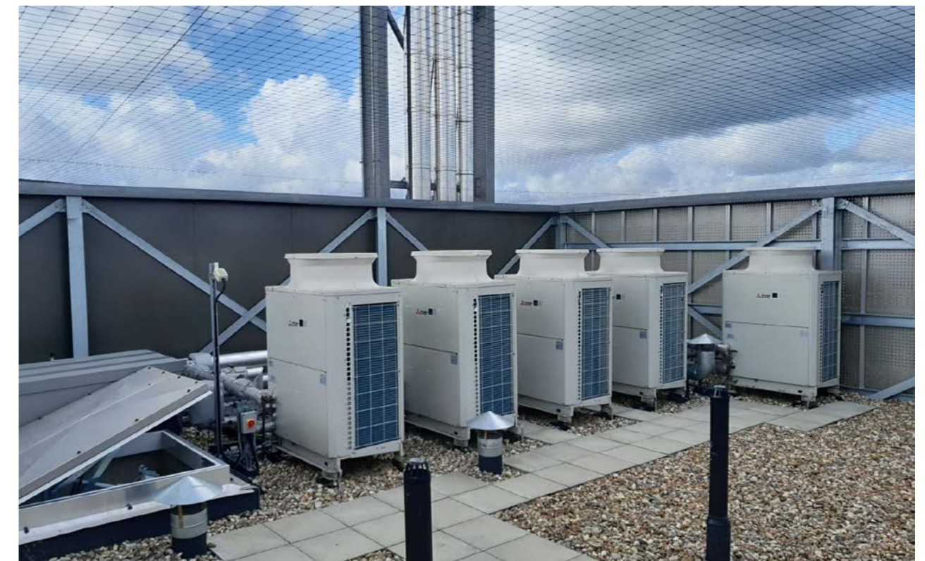
Air source heat pumps at Canalside, Sheerwater
